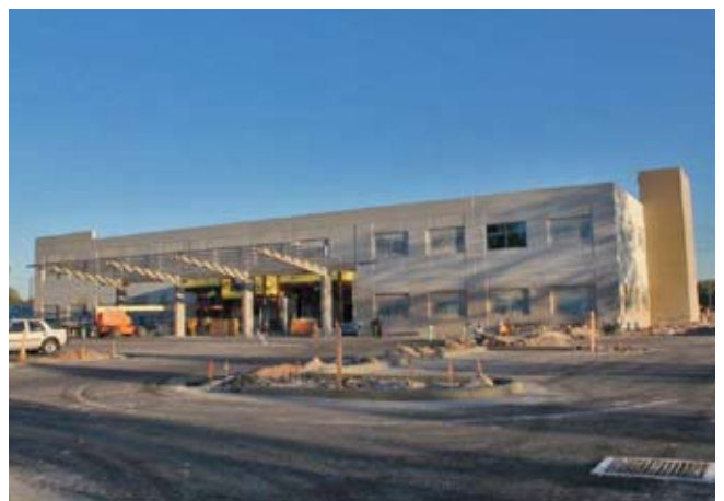
St. Joseph's Hospital - South, Medical Office Building One, River View, Florida for Barton Malow
