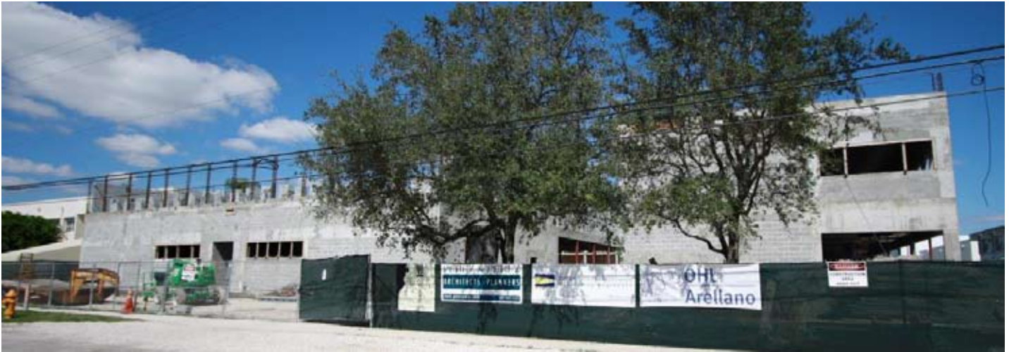
Epiphany Catholic School New Classrooms and School Expansion, South Miami, Florida for Arellano OHL.
